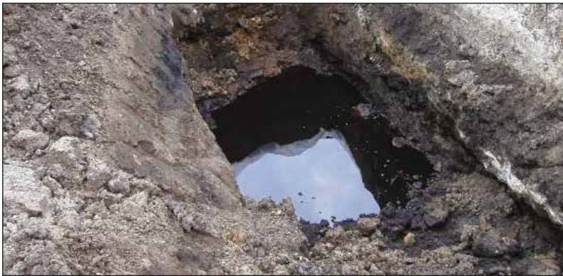
Top Photo: Excavation related to the transaction of a contaminated property, the result of a historic leaking underground storage tank.
